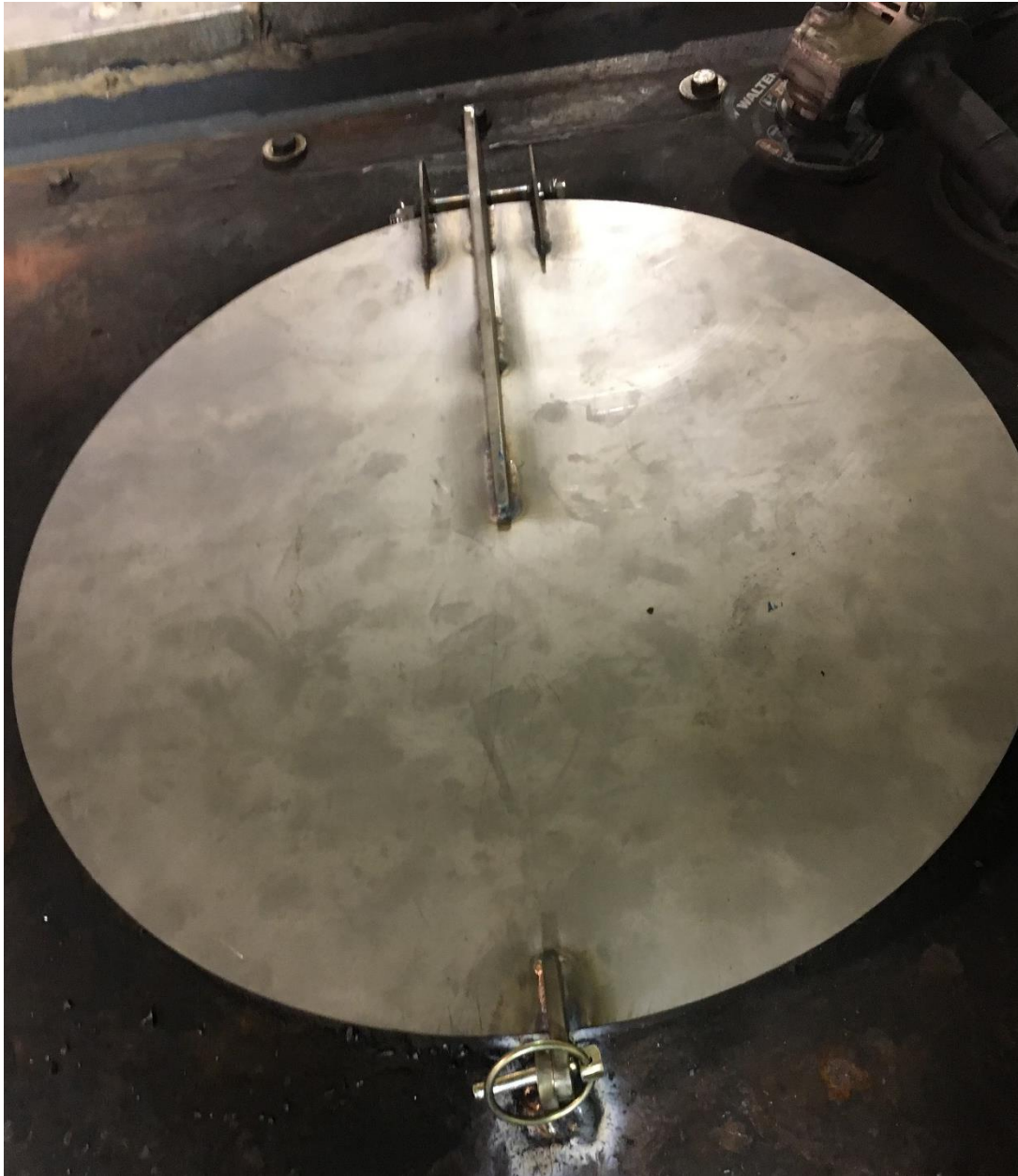
Figure 12 – Exhaust Flap Modified With Securing Latch
