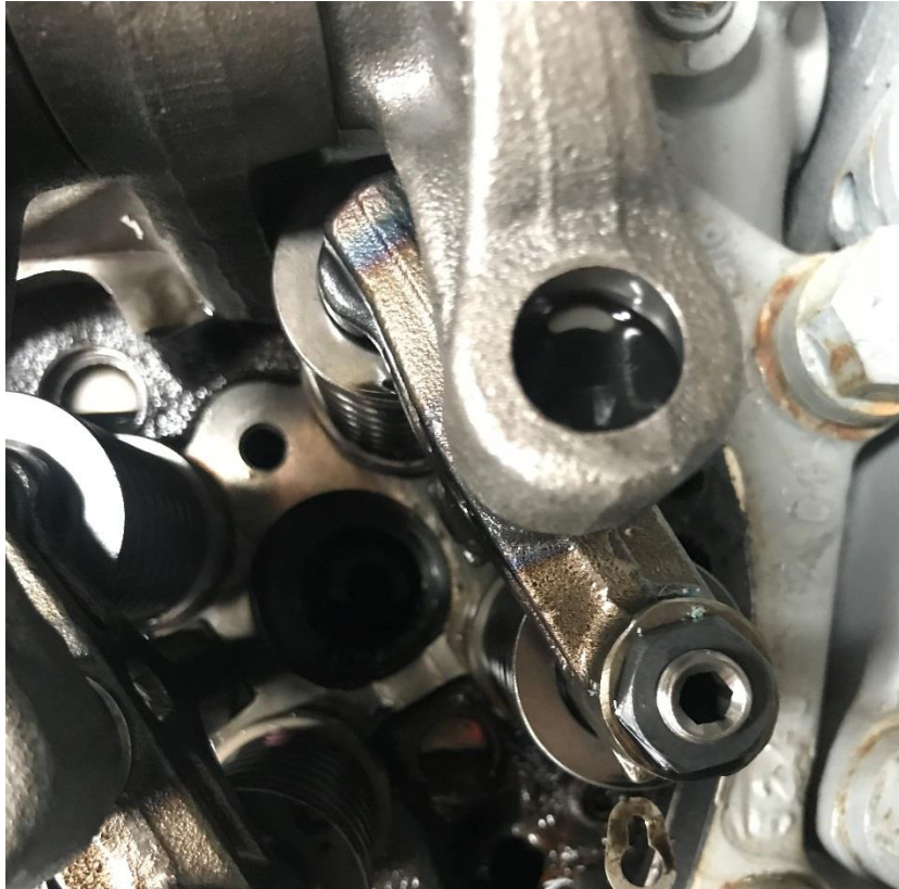
Figure 3 - Water Observed to Top of Cylinder Head
