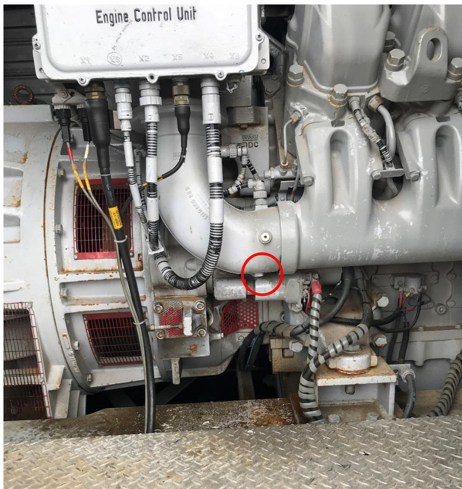
Figure 2 - Intake Manifold. Excess Water was Observed Draining from Condensate Drain.
