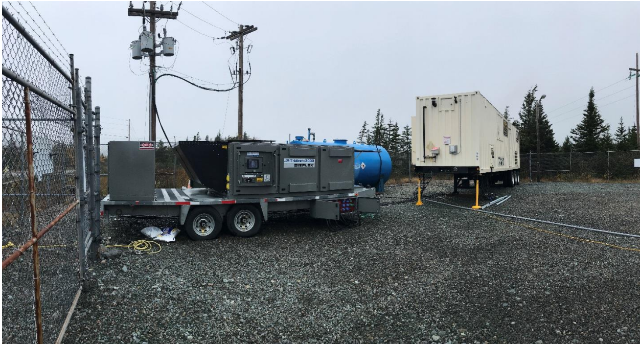
Figure 13 - Rented 2 MW Portable Diesel Generator and Mobile Load Bank Setup in Trepassey Substation
