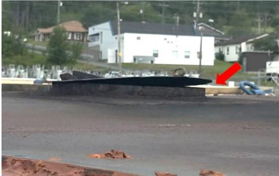
Figure 1 - Damaged/Warped Exhaust Flap
